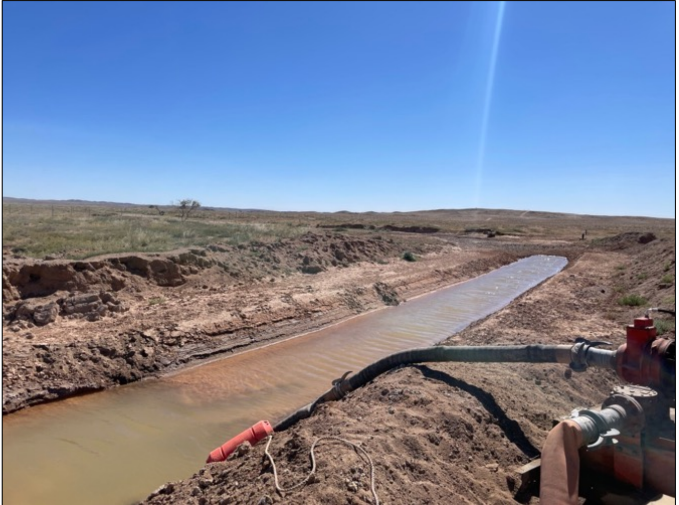
Figure 4-19 Collection of Seepage Water
